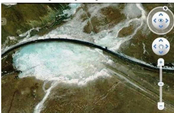
Figure 28. naled threatening railway Naled formed by icing of culvert under Trans-Mongolian Railway, south of Ulaanbaatar. (image: Google Earth - 25 th February 2007)
